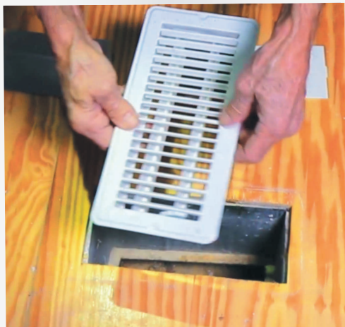
To do: Seal leaky air ducts
