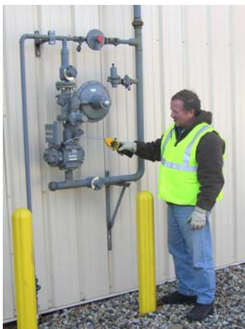
Austin Utilities Gas Service Technician inspecting a commercial gas meter set for leaks.
