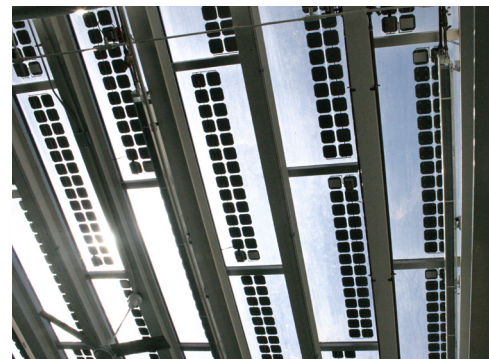
A building integrated solar photovoltaic (BIPV) system installed in the skylights at the Marjorie McNeely Conservatory at Como Park in St. Paul, Minnesota.
