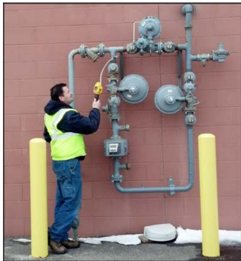
Austin Utilities Gas Service Technician inspecting a commercial gas meter set for leaks.
